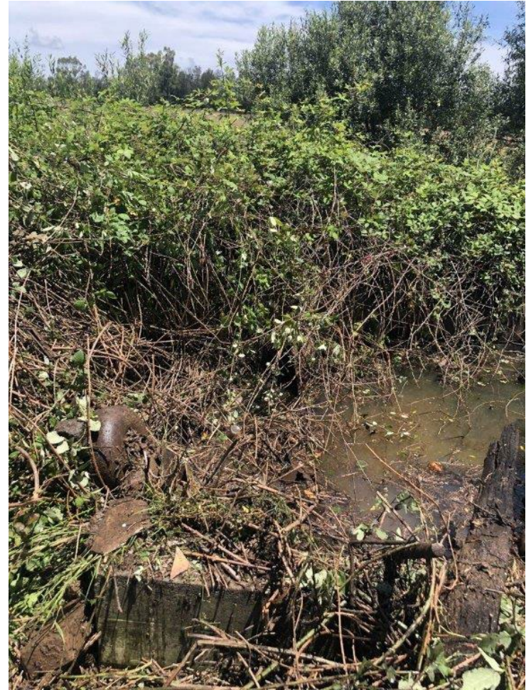
Photo 11: South concrete structure filled with dumped wastes, water and vegetation – AEC 12(S)
